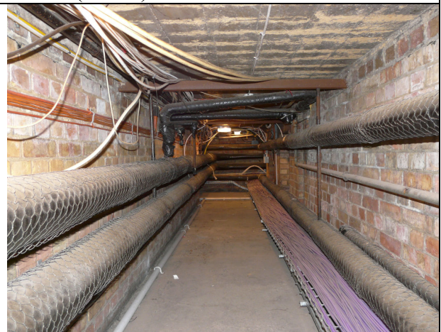
PIPEWORK IN UNDERCROFT (From pump room)
