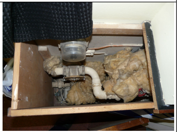
VIEW LOOKING INTO EXISTING ENTRY SERVICE DUCT WITH REDUNDANT CONTROL EQUIPMENT
