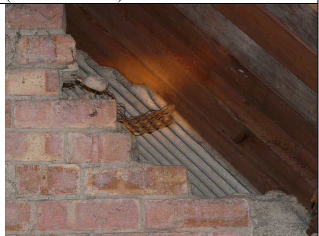
ROOF OVER DINING ROOM SHOWING SECTION OF ABESTOS SHEETING
