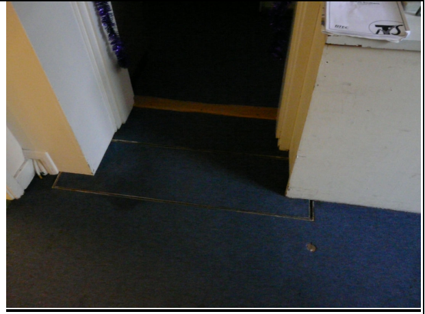
SERVICE DUCT COVER IN FLOOR
