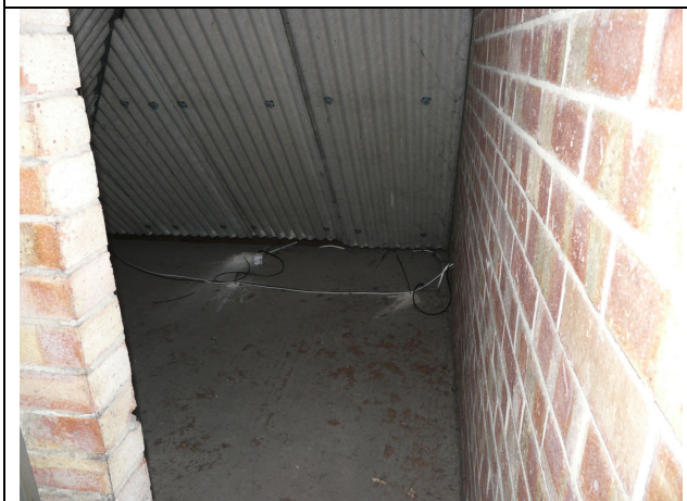
WEST WING ROOF WITH ASBESTOS SHEETING
