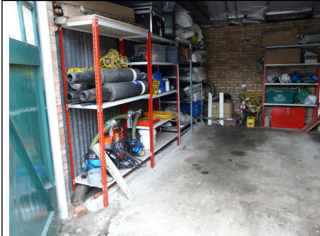
GARAGE WITH GAS METER AND SHOWING GAS MAIN INTO GROUND WITH DENSO PROTECTIVE TAPE
