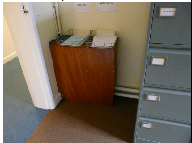
COVER OVER EXISTING HEATING MAIN ENTRY POINT AND CONTROLS ARRANGEMENT
