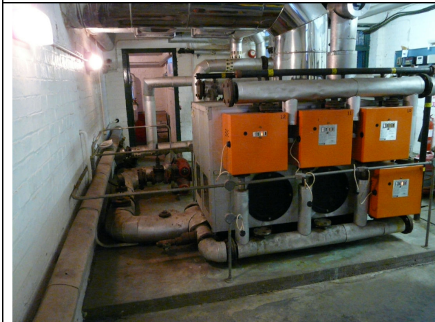
EXISTING BOILER PLANT SHOWING REDUNDANT MODULES AT THE BOTTOM
