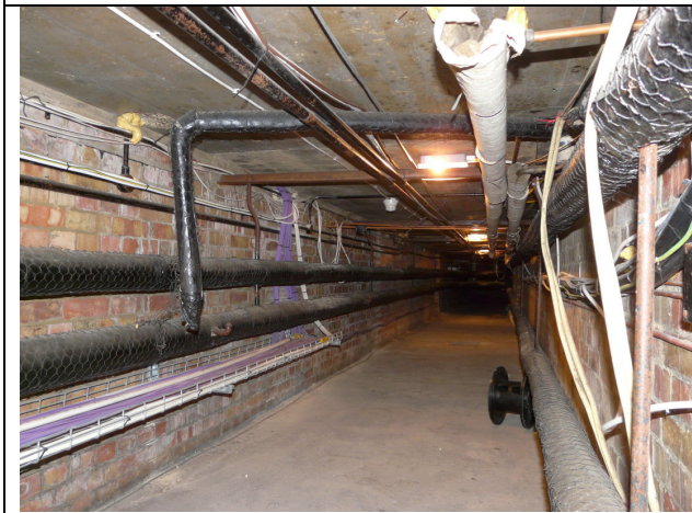
PIPEWORK IN UNDERCROFT (under main corridor)
