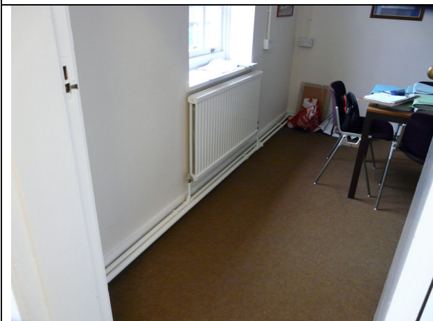
EXISTING PIPEWORK AT LOW LEVEL - UNCASD
